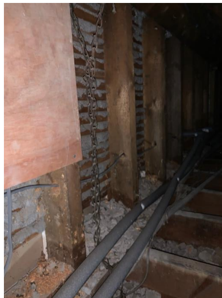
Photo showing the area behind the knee walls of a RIR. Semi-rigid insulation can be friction fitted between the upright timbers and held in place with either a membrane or timber battens.
