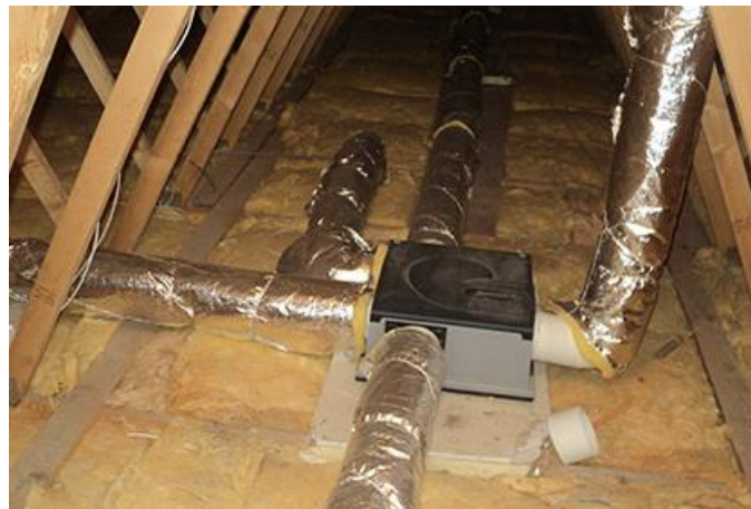
Aereco DCV fan & ducting located in loft. Image: Aereco
