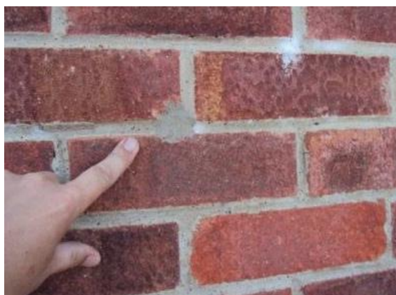
Evidence of CWI
